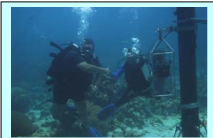
Peter Gayle congratulates his team member on the completion of the installation of the CREWS station.
