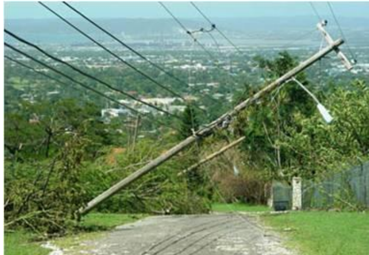
Figure 4.7.1: Hurricane Dean impacts on Public Utilities in Jamaica
