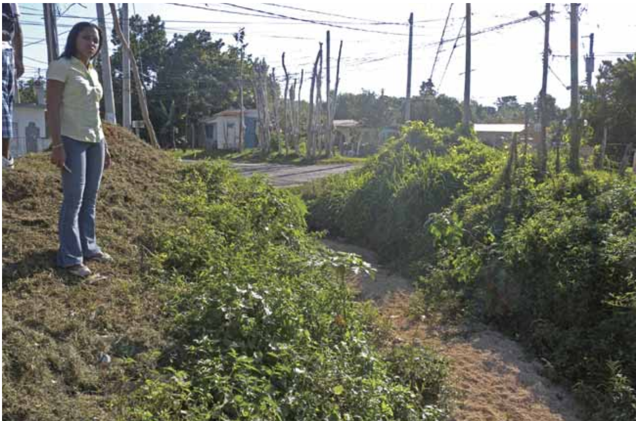
Debris from runoff often clog drainage ways, and natural catchment areas have been partly reclaimed, which exacerbate flooding
