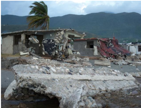
Figure 1. Beach Front Houses Destroyed by Hurricane Ivan Storm Surge on Caribbean Terrace
